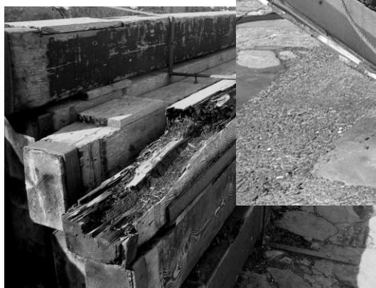
The poor state of the crane and booms.
